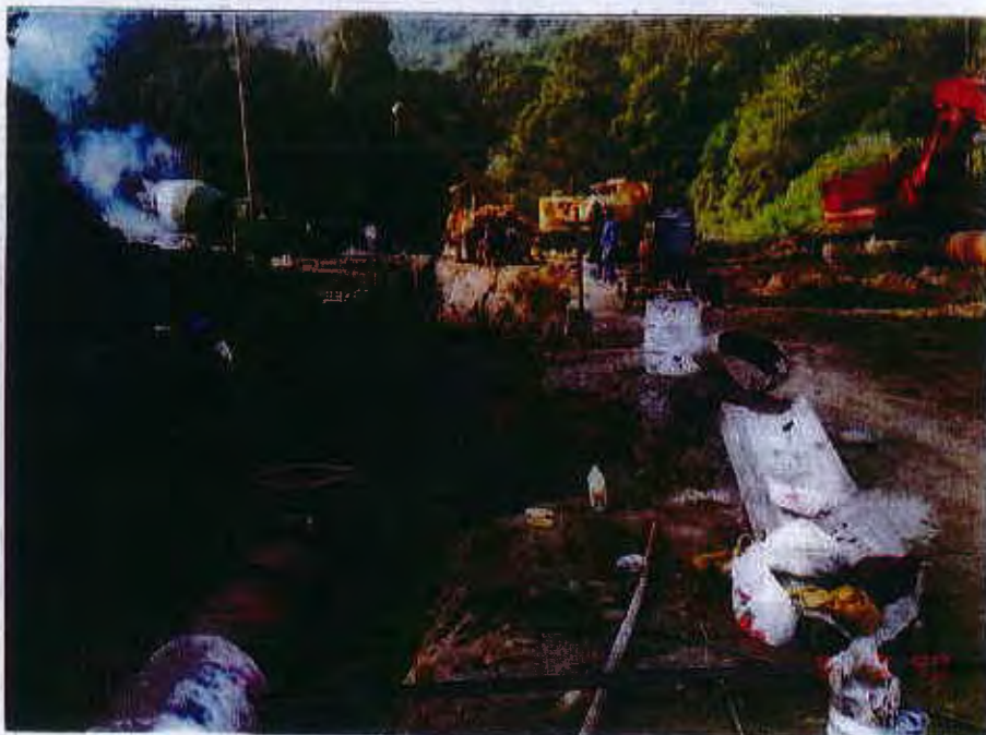
Construction of an access air valve chamber on the 800 mm diameter pipe
