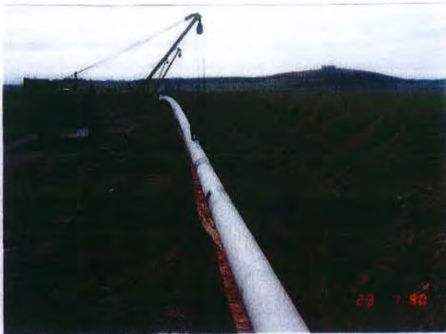
500 mm diameter pipe being snaked into the trench. Mossgas Reservoir on hill on the right.
